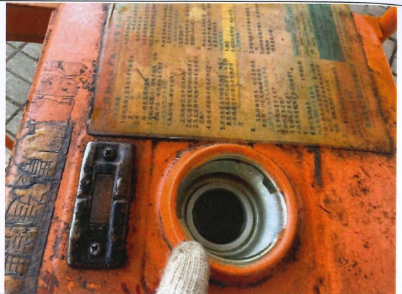
102-S008-02-燃油油位檢查
