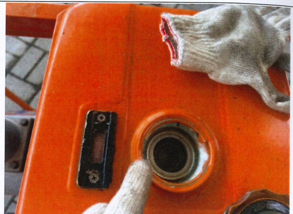
105-S028-02-燃油油位檢查
