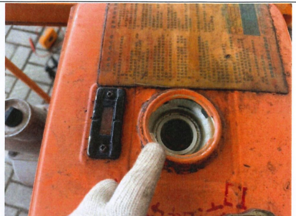
102-S007-02-燃油油位檢查
